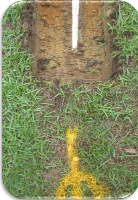
1¼" PVC water pipe at 14" below grade
