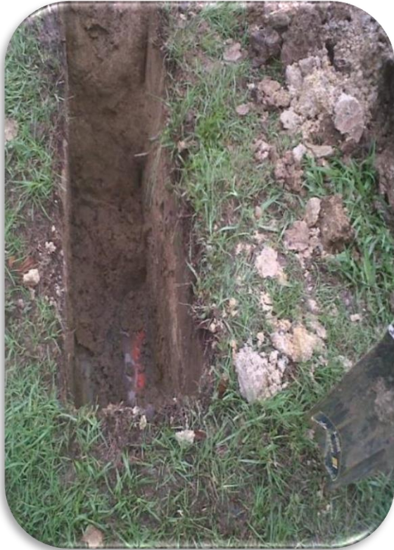
2" PE gas pipe at 42" below grade
